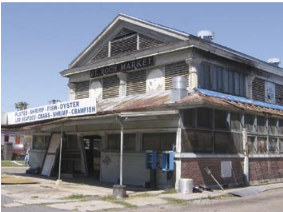
A view of the exterior of the St. Roch Market. Photo by Samantha Bosshart
